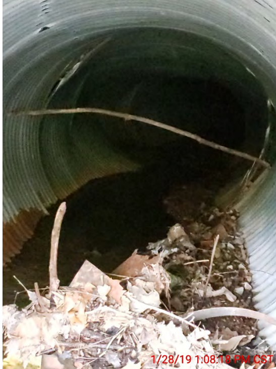
FIGURE 2-26 (AREA 7) INTERIOR OF 54" CMP, DOWNSTREAM OF SCHOOL DETENTION BASIN
