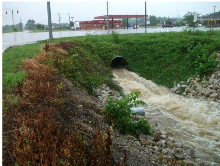
FIGURE 2-47 (AREA 14) 72" CMP – OUTLET SOUTH OF SR 662 (PHOTO FROM JUNE 24, 2013 STORM EVENT)
