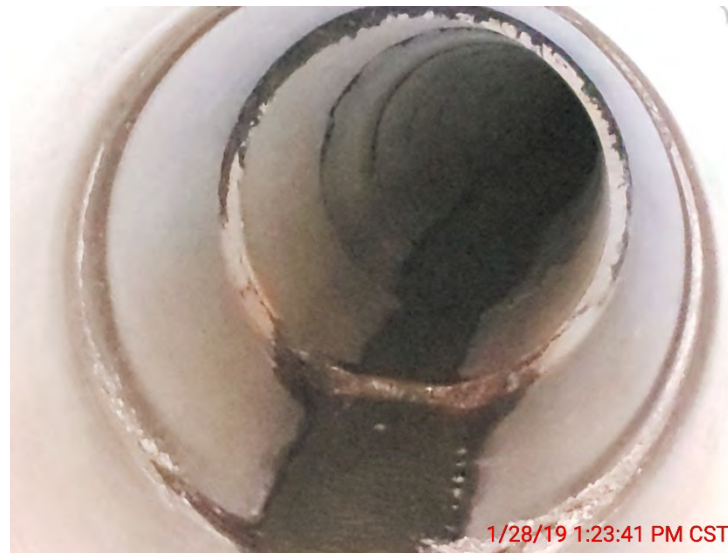
FIGURE 2-21 (AREA 6) EXISTING OFFSET JOINTS WITHIN 60" CONCRETE PIPE CREATING PARKING LOT PAVEMENT SETTLEMENT
