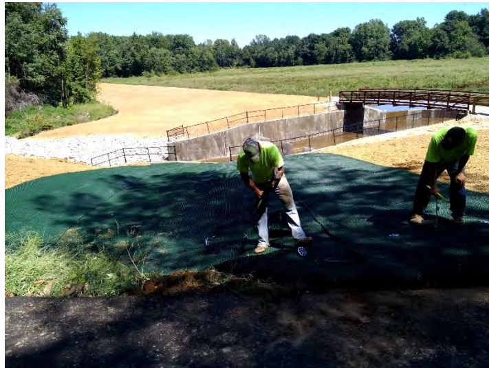
FIGURE 4-1 EXAMPLE OF A HIGH PERFORMANCE TURF REINFORCEMENT MAT FOR A SPILLWAY OVERFLOW; CREWS INSTALLING PERCUSSION GROUND ANCHORS (PHOTO VIA CEI – IDNR WHITE OAK DAM PROJECT)
