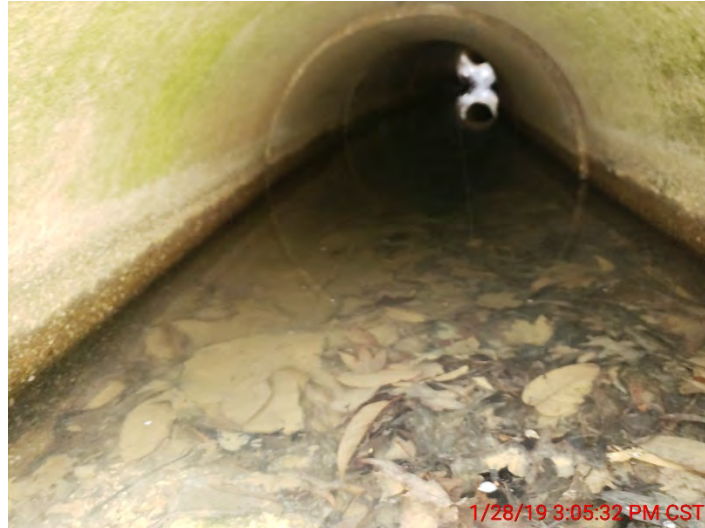
FIGURE 2-15 (AREA 3) 24" CMP HALF FULL OF SEDIMENT
