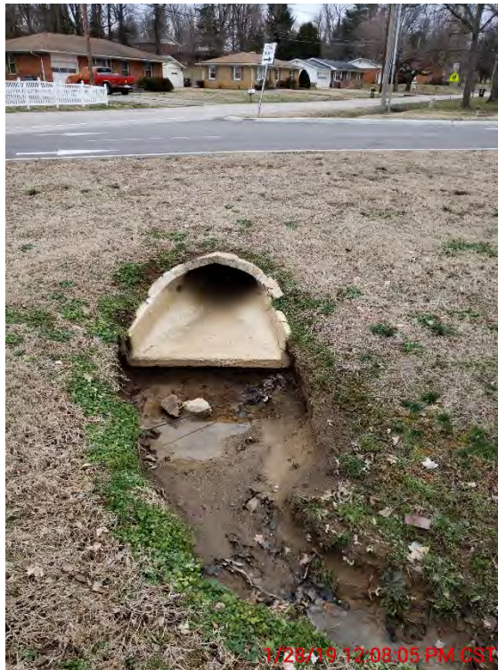
FIGURE 2-39 (AREA 11) EROSION AT 19" X 30" RCP CULVERT OUTLET
