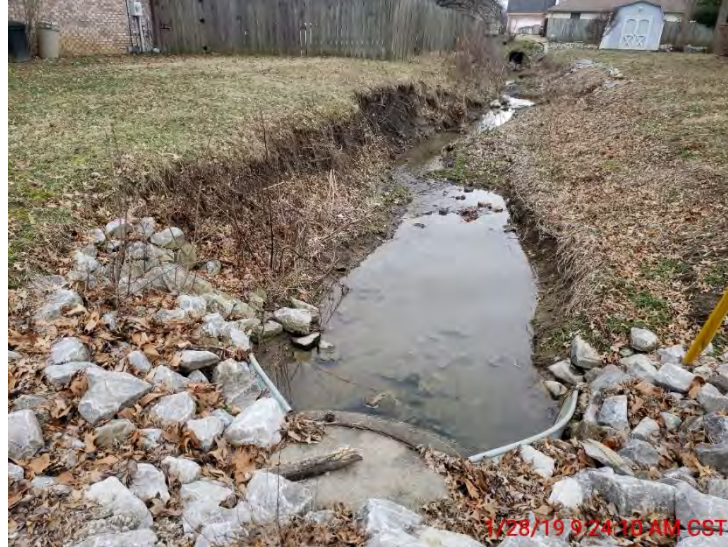
FIGURE 2-42 (AREA 12) ERODING DITCH BANKS WEST OF MAPLE LANE
