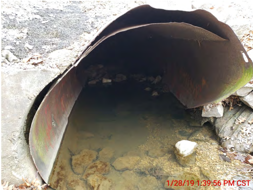
FIGURE 2-23 (AREA 6) DETERIORATION OF 60" STEEL CULVERT AT THIRD STREET
