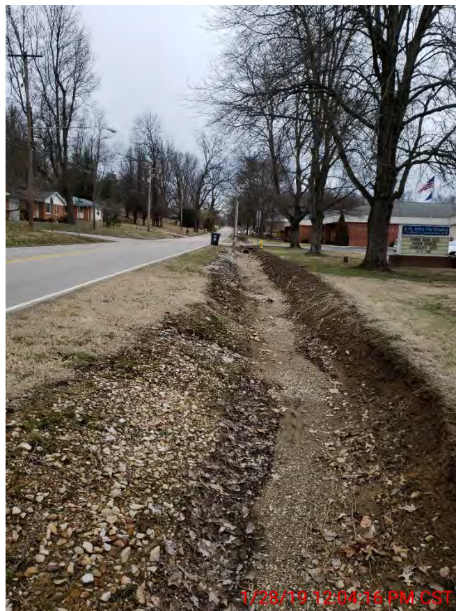
FIGURE 2-37 (AREA 11) OPEN DITCH ALONG FRAME ROAD
