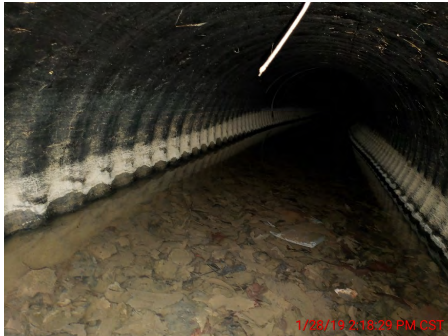
FIGURE 2-19 (AREA 5) MIDDLE STREET 30" HDPE CULVERT WITH SEDIMENT ACCUMULATION
