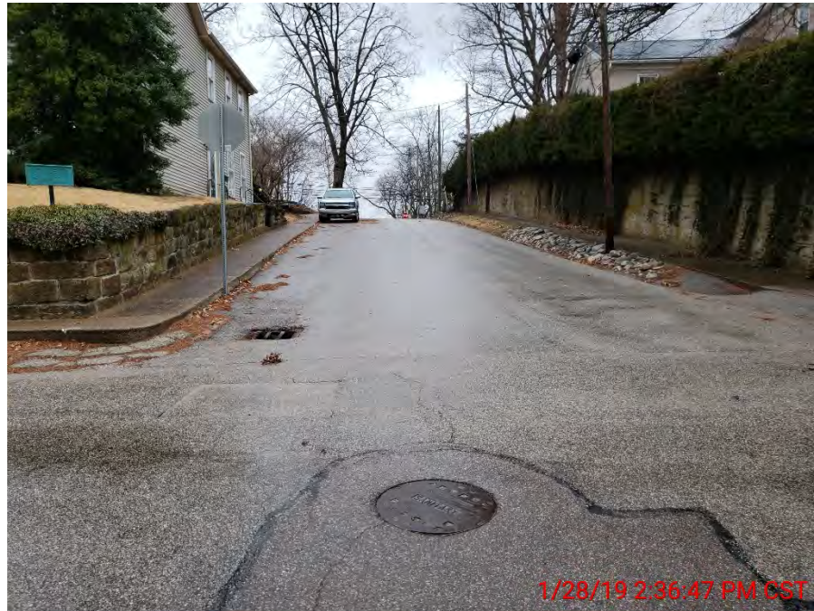
FIGURE 2-17 (AREA 4) STORMWATER SHEET FLOWS DOWN HILL TO RESIDENTIAL PROPERTY
