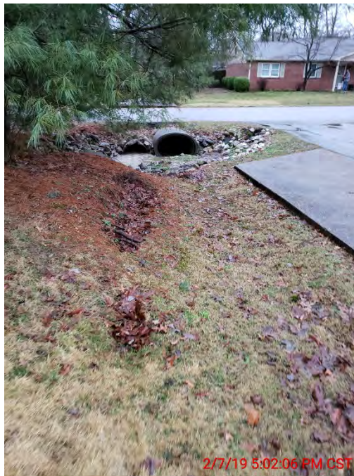
FIGURE 2-4 (AREA 1) EROSION ON WEST SIDE OF FOREST PARK DRIVE, SINKHOLES VISIBLE ABOVE EXISTING 48" CULVERT
