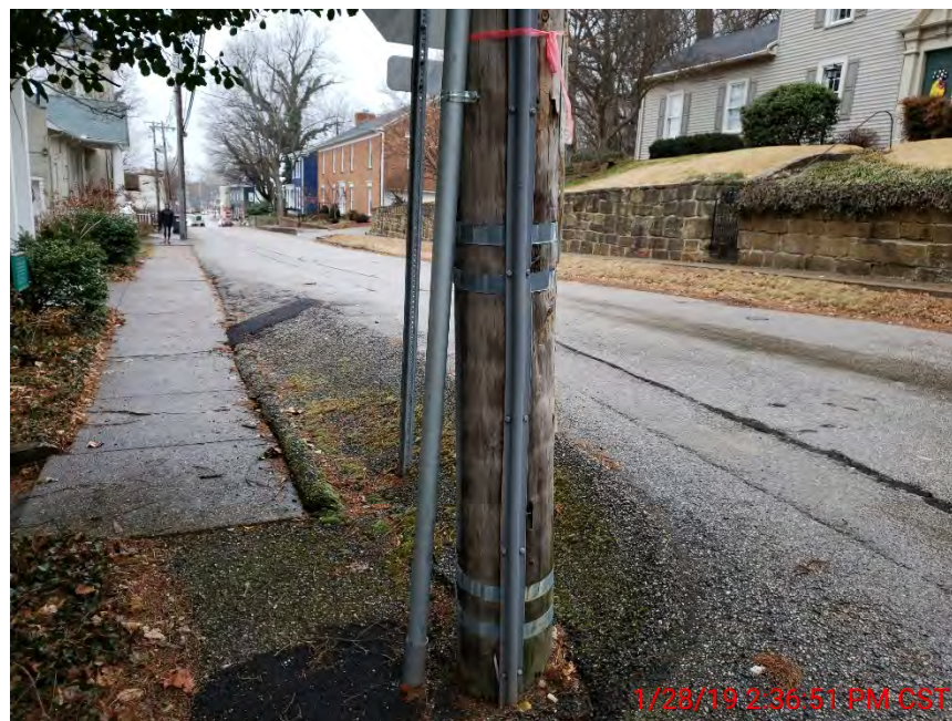
FIGURE 2-16 (AREA 4) ROAD PAVEMENT IS HIGHER THAN SIDEWALK
