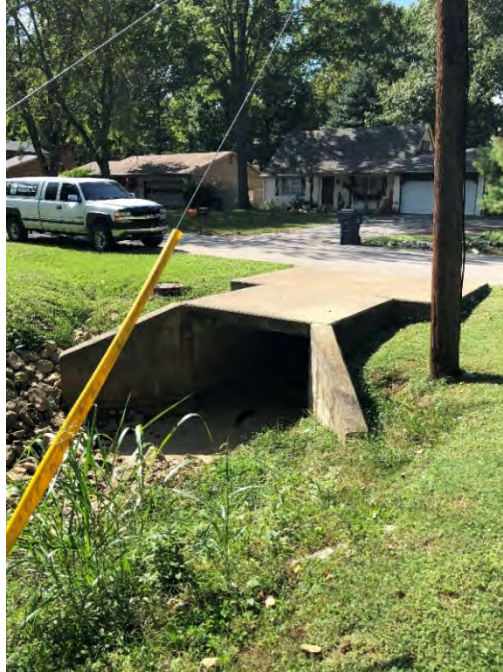
FIGURE 2-3 (AREA 1) 6'X4' BOX CULVERT ENERGY DISSIPATION FACILITY AT FOREST PARK DRIVE OUTFALL
