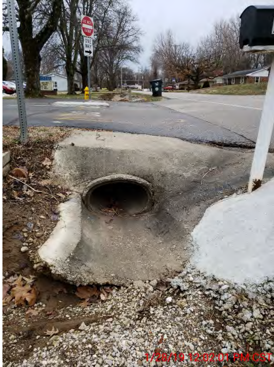
FIGURE 2-38 (AREA 11) EROSION AT 14" X 23" RCP CULVERT INLET AT SCHOOL ENTRANCE
