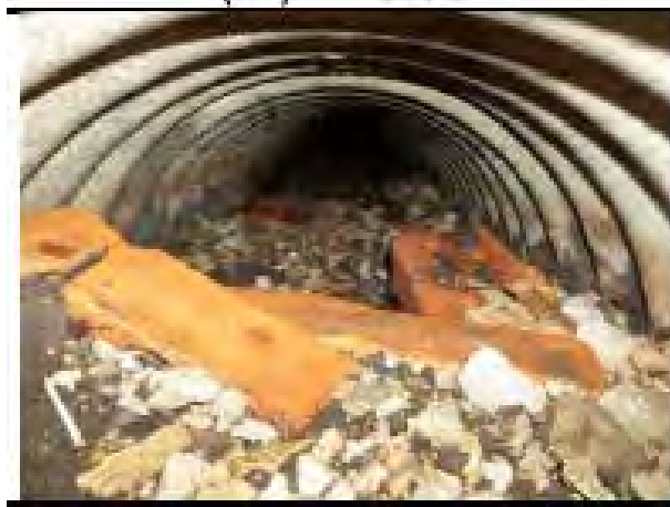
FIGURE 2-30 (AREA 8) CULVERT AT MADISON AND JENNINGS STREET, FULL OF SEDIMENT (PHOTO FROM 2015 JENNINGS STREET CORRIDOR STUDY)
