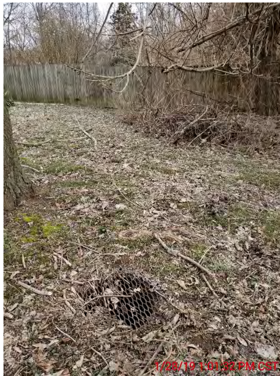
FIGURE 2-27 (AREA 7) SINK HOLES NEAR INLET SOUTH OF FIRST STREET
