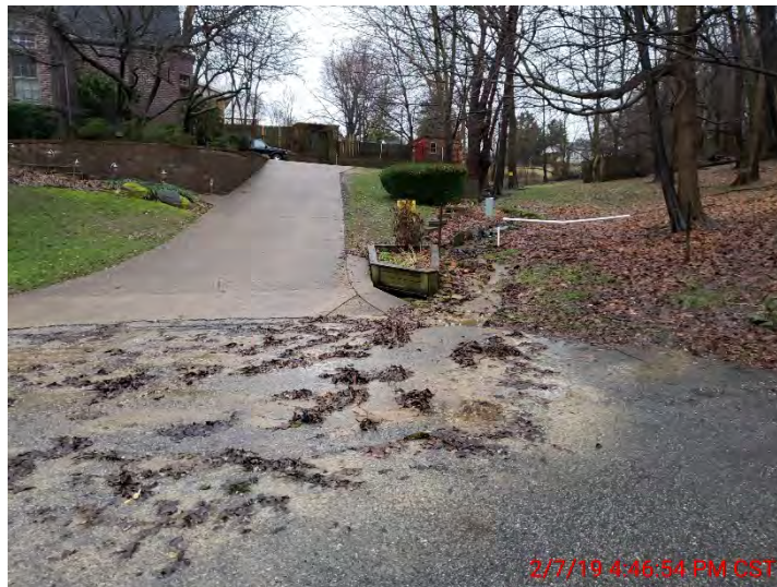
FIGURE 2-13 (AREA 2) CONCENTRATED FLOW AT DEAD END OF CUL-DE-SAC ENTERING ROAD
