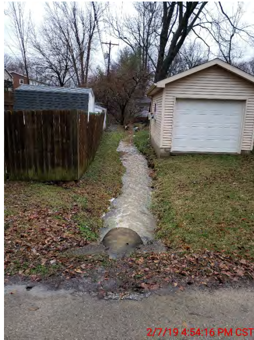
FIGURE 2-7 (AREA 1) 21” RCP CULVERT UNDER TREELANE DRIVE WITH GARAGE FOUNDATION EROSION IN BACKGROUND
