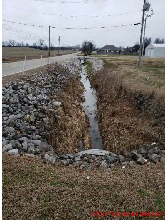
FIGURE 2-46 (AREA 14) ELLERBUSCH OPEN DITCH WITH STEEP DROP OFF AT CASEY'S GENERAL STORE
