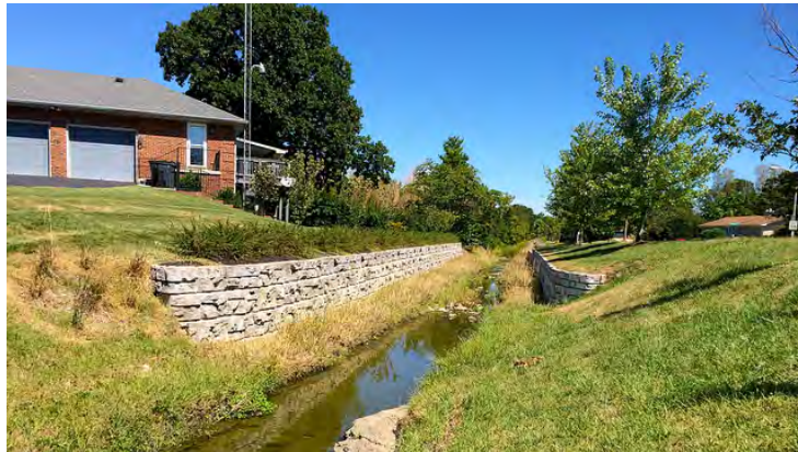
FIGURE 4-3 EXAMPLE OF LARGE PRECAST BLOCK WALL LINING CHANNEL WITHOUT STEP BACK (PHOTO VIA REDI-ROCK)
