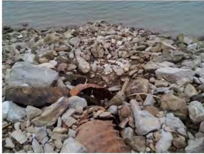
FIGURE 2-29 (AREA 8) MONROE STREET OUTLET – SEVERELY DETERIORATED AND BURIED (PHOTO FROM MS4 – 2015 OUTFALL RECONNAISSANCE REPORT)
