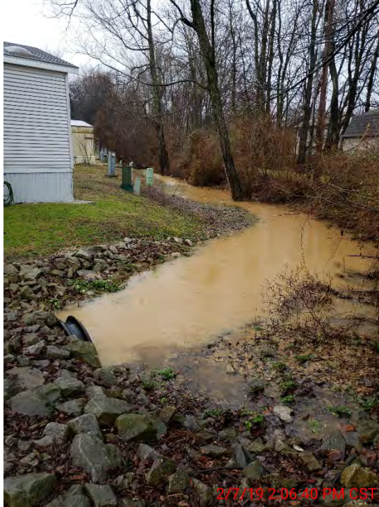
FIGURE 2-40 (AREA 12) 36" HDPE OUTLET AT LOWER KNOB HILL DRIVE
