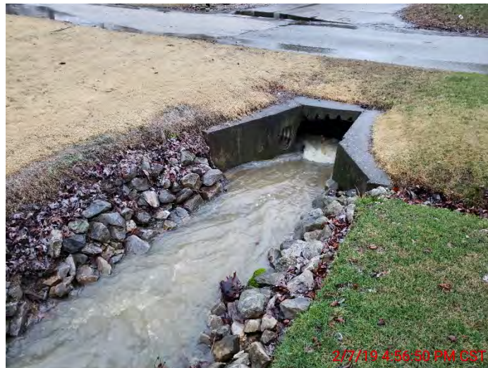
FIGURE 2-6 (AREA 1) 30" HDPE, WITH 15" CMP OVERFLOW, ACROSS TREELANE DRIVE
