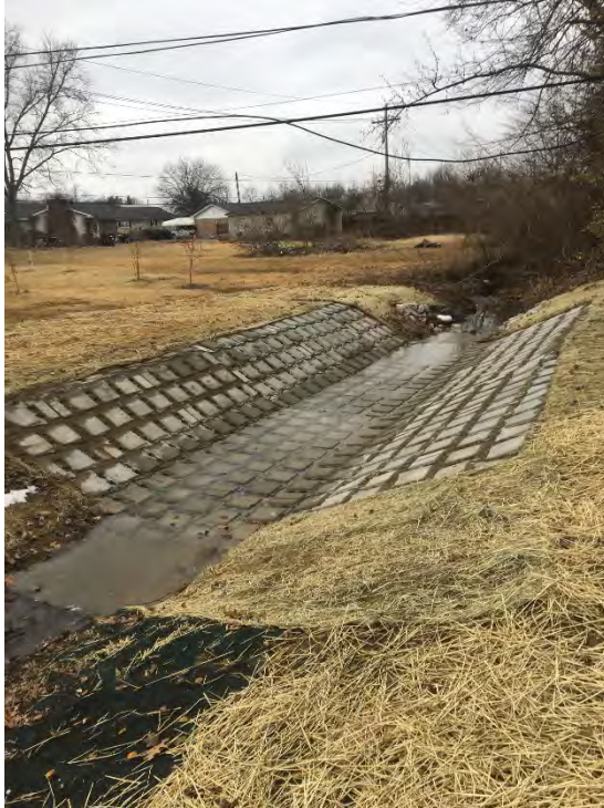
FIGURE 4-2 EXAMPLE OF ARTICULATED CONCRETE BLOCK MAT SYSTEM INSTALLED IN UNNAMED TRIBUTARY TO SUMMER PECKA DTICH NORTH OF LINCOLN AVENUE (PHOTO VIA CEI – TOWN OF NEWBURGH SANITARY SEWER PROJECT)
