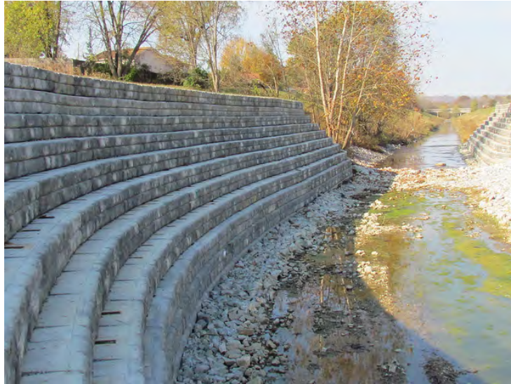
FIGURE 4-4 EXAMPLE LARGE PRECAST BLOCK WALL LINING CHANNEL WITH STEP BACK (PHOTO VIA REDI-ROCK)
