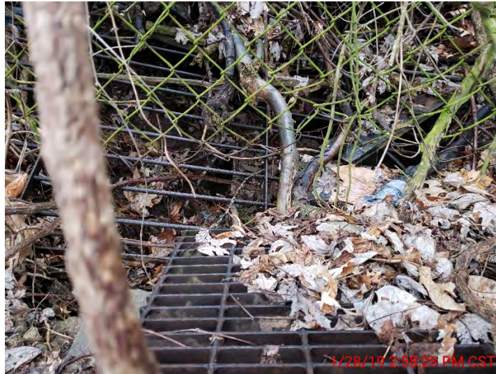
FIGURE 2-14 (AREA 3) DEBRIS COVERED INLET ALONG 24" CMP
