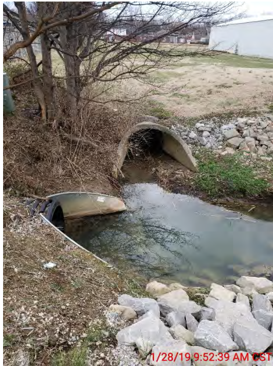
FIGURE 2-45 (AREA 14) WINDSOR POINT 42" OUTFALL (FRONT) AND EXIST 36" HDPE CULVERT ACROSS SOUTHGATE BLVD. WITHIN ELLERBUSCH DITCH
