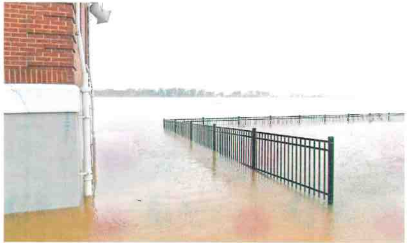
Ohio River flood waters surround the old U.S. Lock and Dam in Newburgh.
