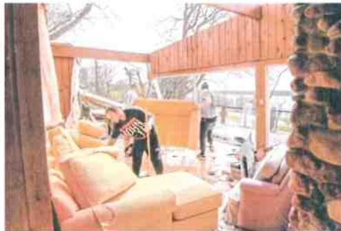
Workers with Waggenheim Moving and Handling clear a room at 421 East Jennings as utility crews, homeowners, moving companies and customers help clean up and restore order on Monday. PHOTO BY JAMES GIBSON
