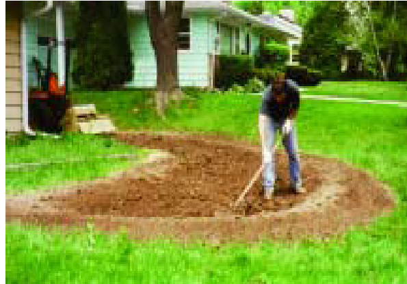
On a gentle slope, soil from digging out the garden can be used to create the berm. This rain garden is 4” deep.
